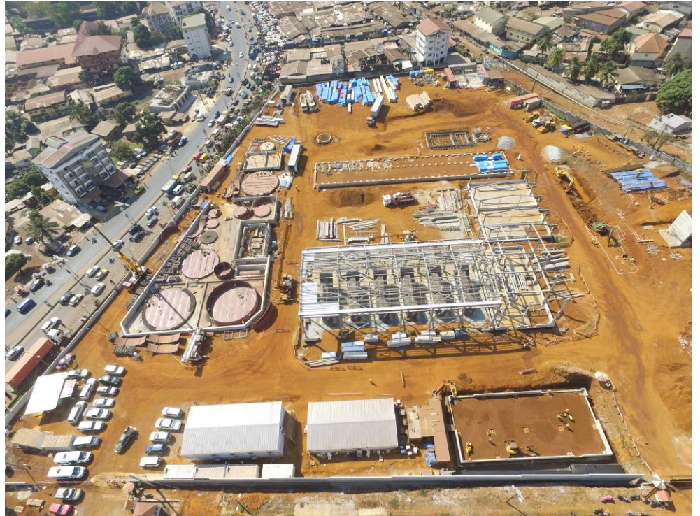
MAN Energy Solutions installs six MAN 18V32/40 engines with a total capacity of 53 MW in a power plant in Conakry, Guinea.
