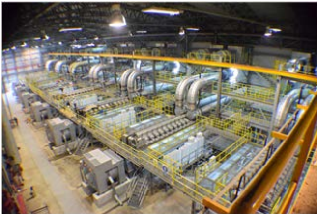
Seven MAN 32/44CR engines provide around 78 MW of electrical energy
